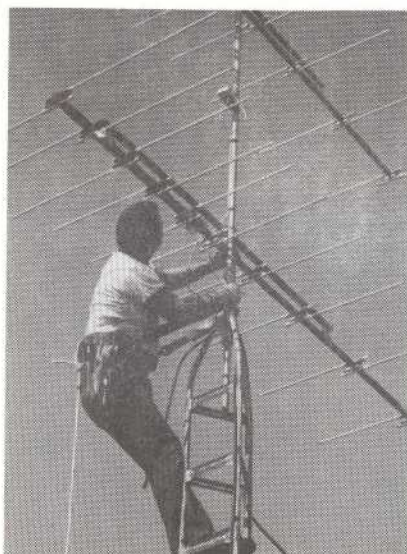
Rabong orients both antennas so they point directly to reception area desired.
