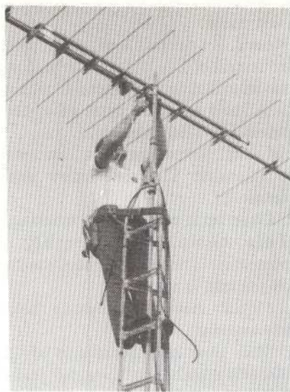
Rabong attaches the top antenna to the mast, tightening down the U-bolt securely.
