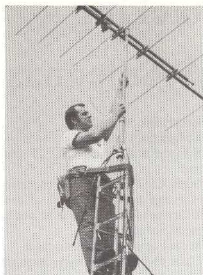
The CC-787 coupler is mounted approximately 36 inches below the upper antenna.
