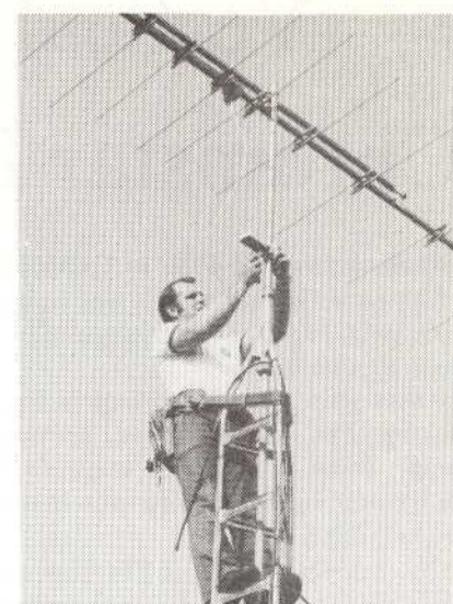
After connecting the cable from the upper antenna to the "set 1" jack of the CC-787, Rabong connects cable from housing bottom of lower antenna to "set 2" jack of coupler.
