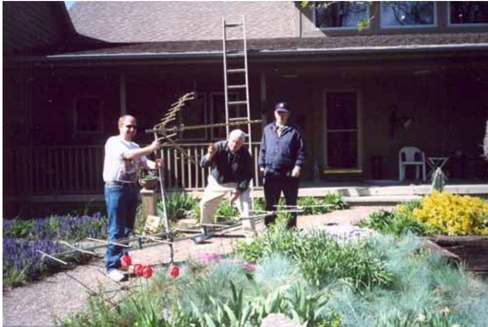
Fybush, Lucas and Bond getting FM and UHF antennas ready for Jim's roof. (5/12/07)
