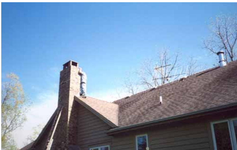
Bonding with chimney that will soon be stopped by antenna placement.
