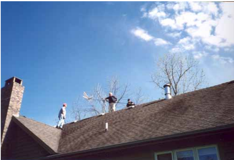
Renfrew, Lucas and Bond pass it on! Note: Fybush on the ground during entire installation.
