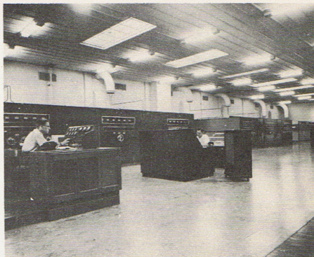
Radio Australia's Transmitter Hall at Shepparton, Victoria. Incoming programs from Melbourne for VLA, VLB, and VLC transmitters are controlled by a technician at the master panel (left).
