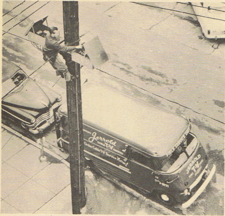
By-passing distribution amplifier with stand-by amplifier in truck permits complete on-pole test of working equipment. Equipped with two-way radio, full test bench, and an emergency power supply; this Dubuque (Iowa) Jerrold CATV system truck is ready for trouble calls anywhere.
