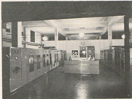
The Transmitter Hall of the British Broadcasting Corporation (BBC) shortwave station at Rampisham. The Hall contains 4 high-powered transmitters and was divided into two by a wall as a precaution during World War II.
