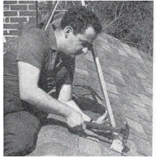
START MOUNTING BOLTS with a hammer. Be sure they are going into the rafters for a firm solid grip. Cover with silicone rubber or tar to prevent leaks.
