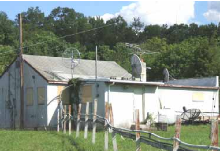
The abandoned WNNJ-1360/103.7 studio and transmitter building. There's a bunch of dead & obsolete stuff in here, and a bunch of bumper stickers.
