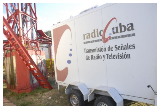
One of Radiocuba's engineering service trailers at the San Isidro Ilegó antenna park south of the city of Sancti Spiritus.
