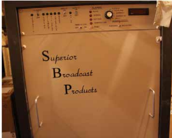
Exhibit 2 - KCOS-LP Inoperative Analog UHF Channel 28 TV Transmitter
